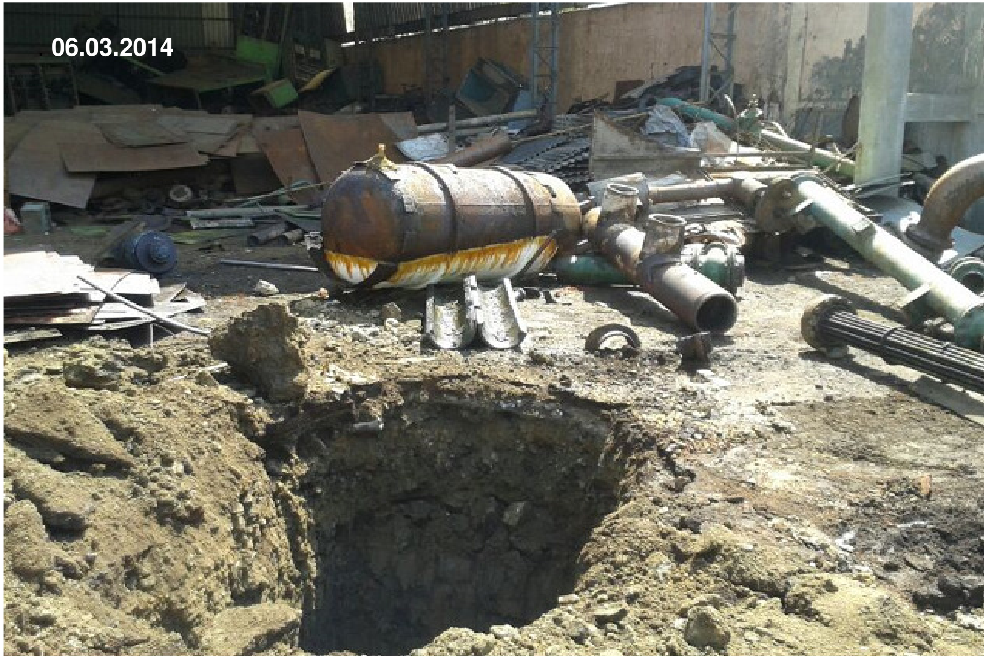
A pit was dug near leaking cylinder on 6th March to attempt Neutralization of Chlorine gas The cylinder that was pegged on earlier night. the ice formation on cylinder may be seen
